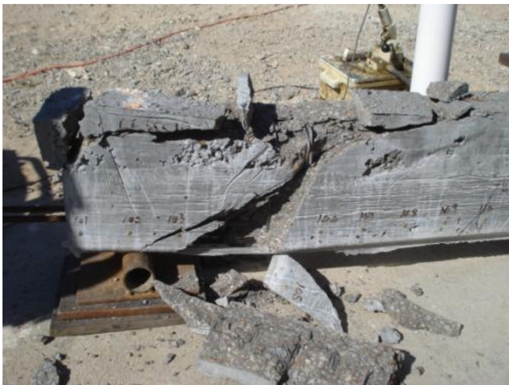
Figure 6.63: Shear failure of specimen HSC-3L
