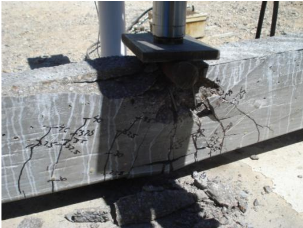
Figure 6.58: Cracking and failure of specimen HSC-2D
