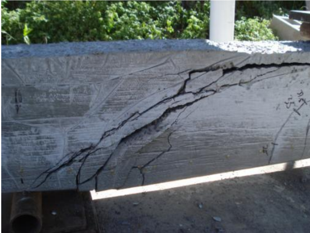
Figure 6.69: Shear cracking of specimen HSS-1D
