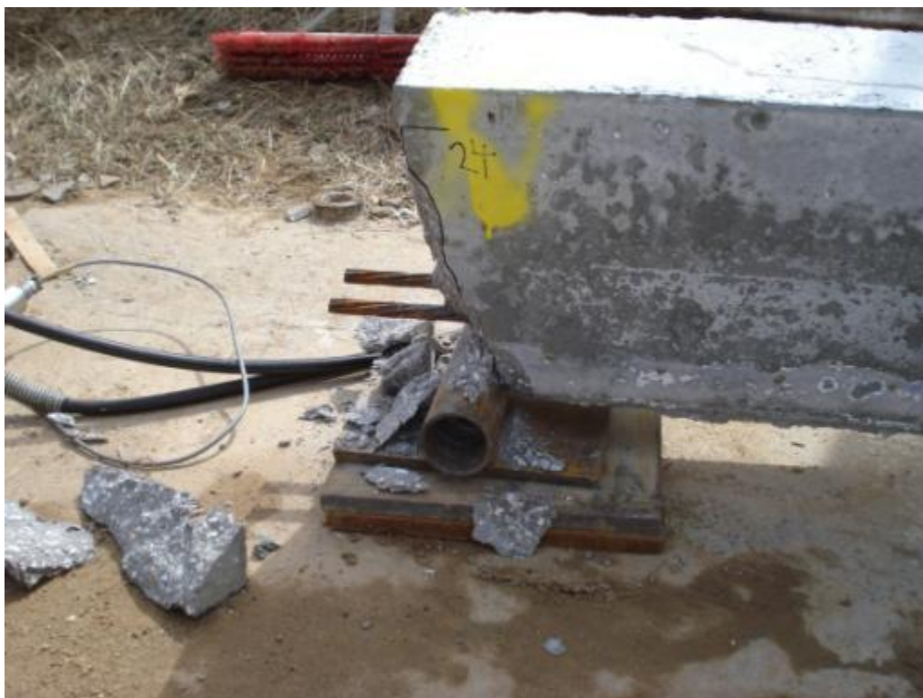
Figure 6.42: Spalling at support of specimen NSL-2D
