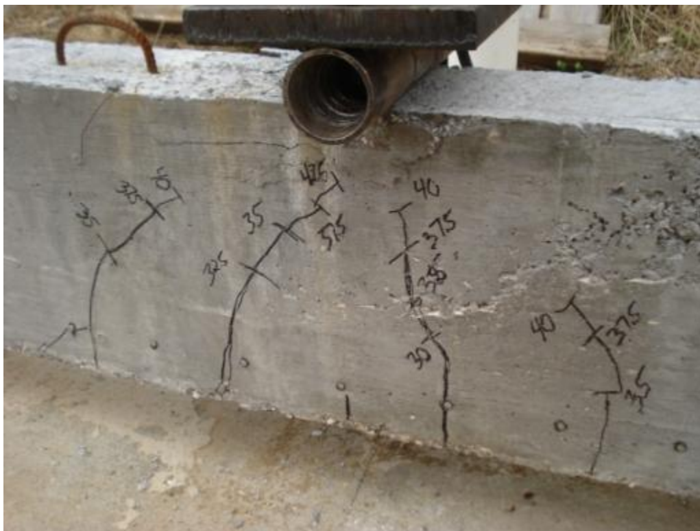
Figure 6.51: Cracking and failure of specimen NSL-4L
