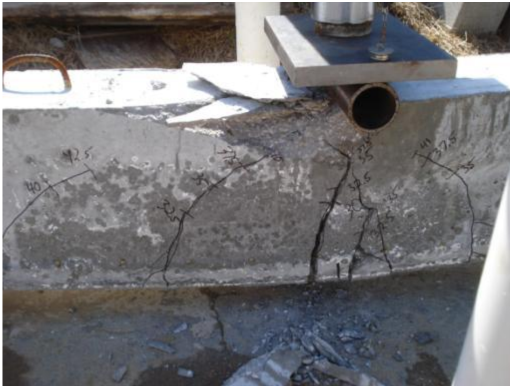
Figure 6.43: Cracking of specimen NSL-2L
